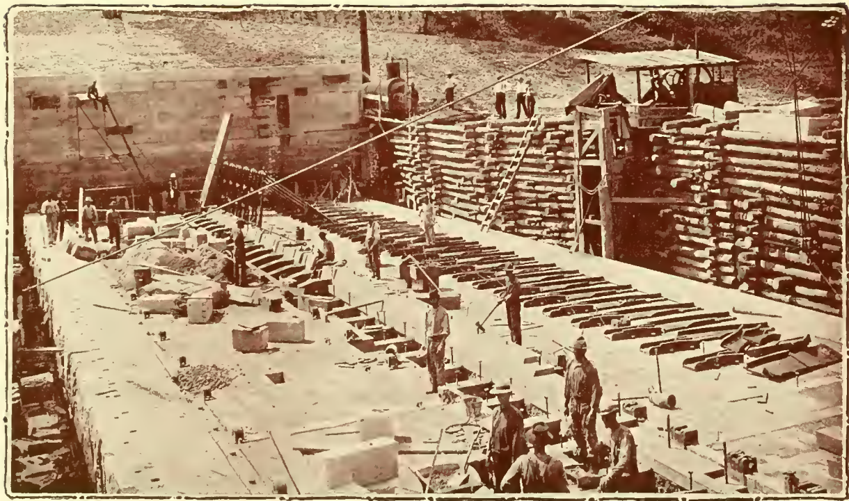
Lock and Dam No. 6, four Miles below Charleston. View of part of the Dam (the "Navigation Pass" part) during construction. Inside of the coffer dam next to the lock. The foundations of this part of the work are shown nearly completed. One wicket and one bridge trestle are standing in place next to the lock wall. Several wicket horses and props, ready to receive the wickets, are also erect in place. Other irons, as hurters, trestle boxes, &c., also partly placed.
